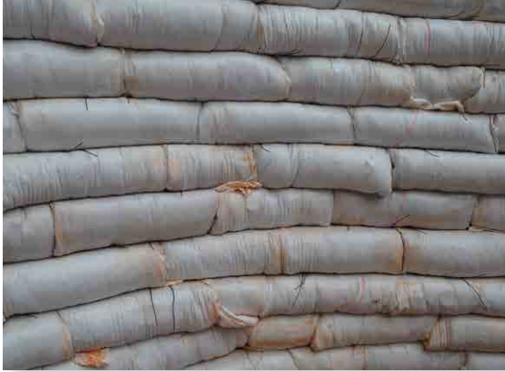
Figure 10. Notice the running bond and vertical seams as well as tie wires sticking out between courses. The hanging brick held barbed wire into place until displaced by an earthbag; string aids in keeping the bricks near the working level of construction instead of having to place and pickup bricks
