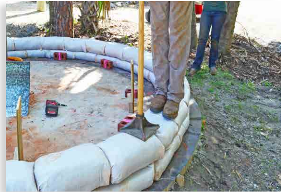
Figure 7. After all bags in a course are in place, tamping flattens, levels, and sets the bags.
