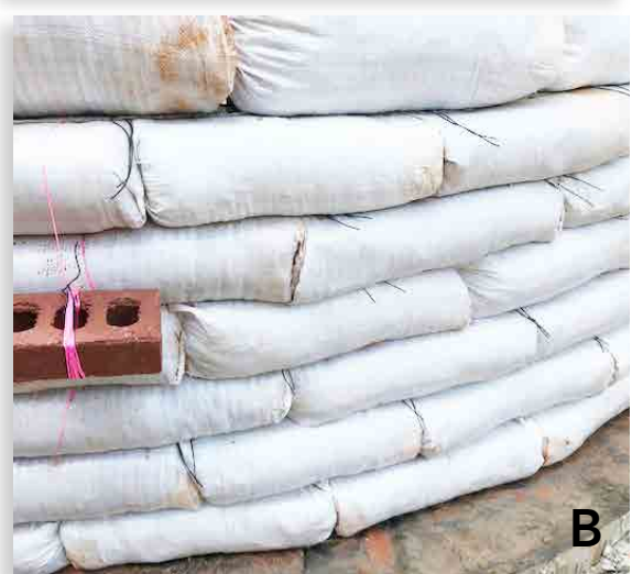
Figure 6. (A) Sliding an earthbag into place using a slider. Notice that bags are placed firmly against one another. Staff member, Elliott Toevs, is also diddling the corners before moving on to the next bag. (B) Notice vertical seams, important for ensuring structural integrity of earthbag structures.
