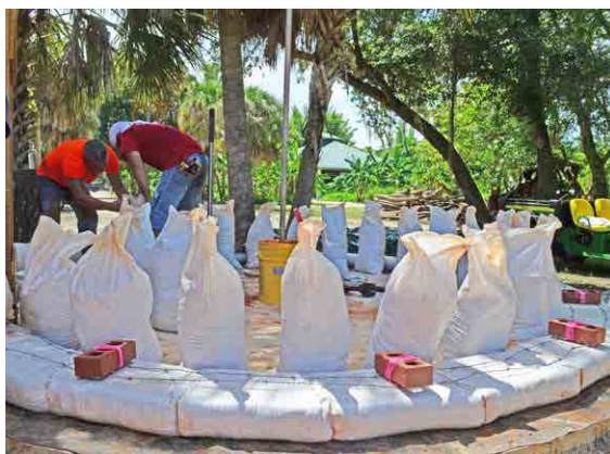
Figure 5. Filled bags are placed along the perimeter of the coursework in preparation of placement. Note the pole in the orange bucket, used in combination with a string to place each bag the same distance (circle radius) from the center of the structure.
