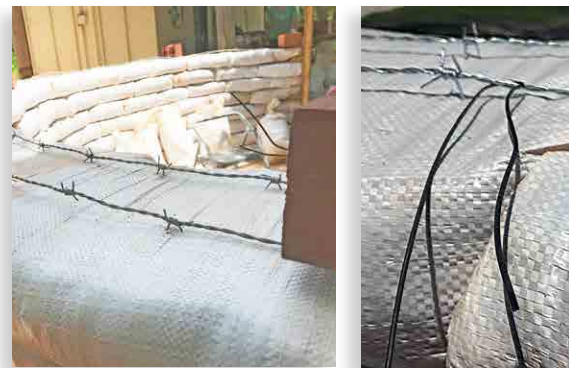
Figure 8. Close-up of barbed wire (top) and tie wires (right) atop tamped earthbags. Bricks hold the barbed wire in place as the next course is laid.
