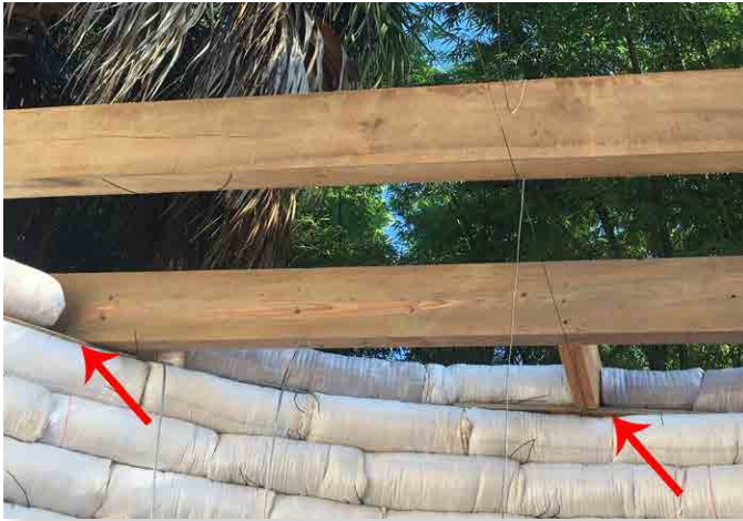
Figure 12. Ceiling joists and a rafter tie are worked into the fourth course from the top at ECHO Florida's location. Source: Tim Motis.
