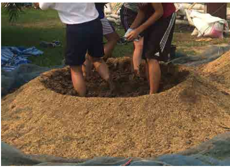
Figure 11. Mixing plaster to cover the walls of an earthbag house. Source: ECHO Asia staff
