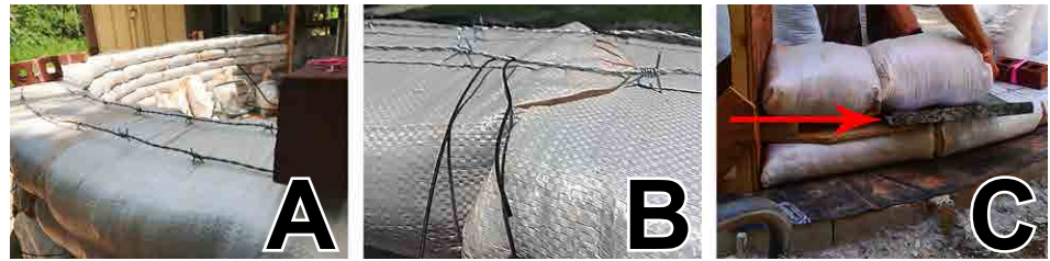
Figure 8. Barbed wire (A) and rebar tie wire tied to barbed wire (B) for interlocking earthbag wall components. Photo C shows a piece of sheet metal used to prevent bags from catching on the barbed wire during placement. Source: Cody Kiefer
