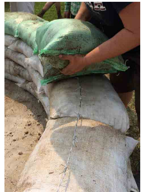
Figure 5. Placing an earth-filled bag on earthbag house wall. Source: ECHO Asia staff
