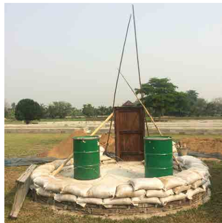
Figure 4. Foundation of earthbag house at ECHO in Asia. Source: ECHO Asia staff
