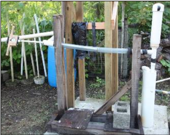
Rower pump with 27' suction pipe in borehole
