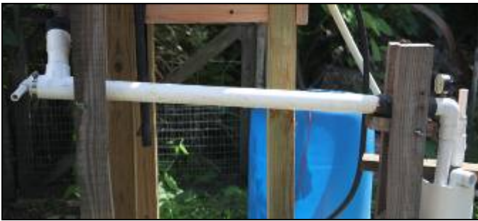
Rower pump installed at a borehole
